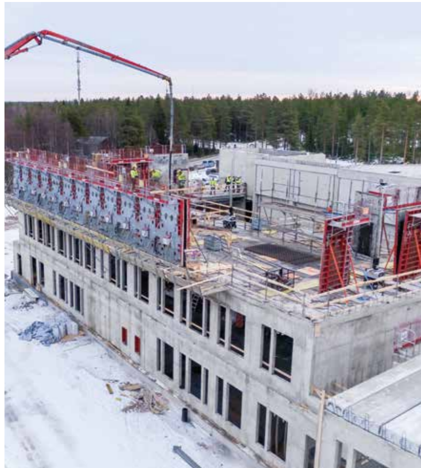
Concrete should not be colder than 5° C. With the temperature sensor, the concrete can be monitored in real time during the cold season – also from the comfort of the office.
