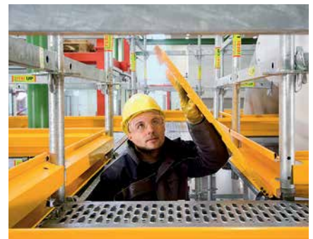
Hatches painted in a yellow signal colour can be opened in a sideways direction. They close automatically which eliminates any source of danger.
