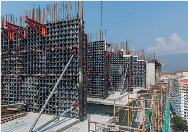
Successful first use of the lightweight system formwork for the construction of shear walls.
