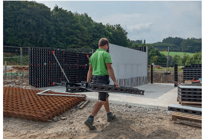
"Formwork newcomers" from the gardening and landscaping sector use DUO for forming bulk material containers.
