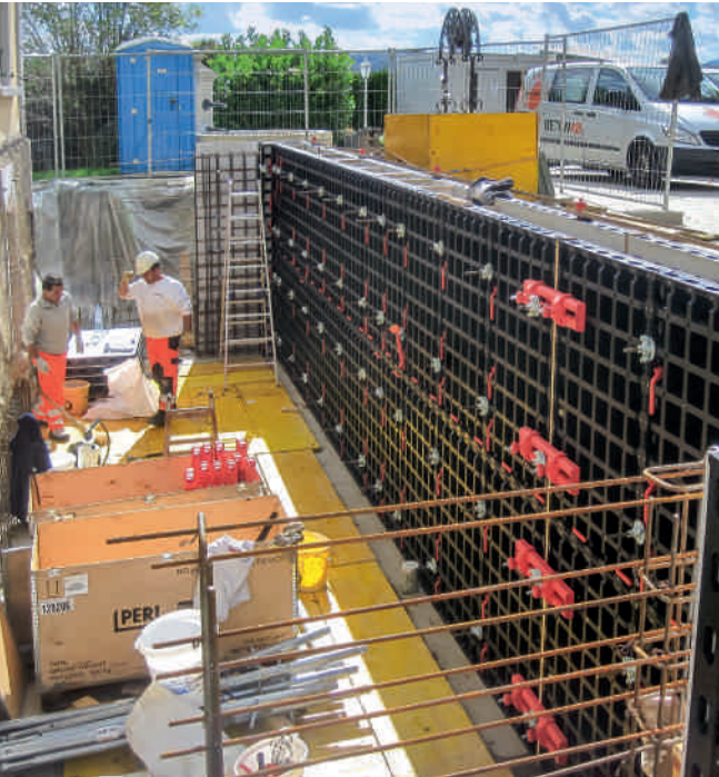
Modifications and extensions without the use of a crane – best solved with DUO.
