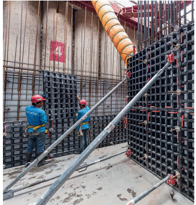
Low weight, small-format formwork elements – DUO showed off these advantages to the full with these basement walls.
